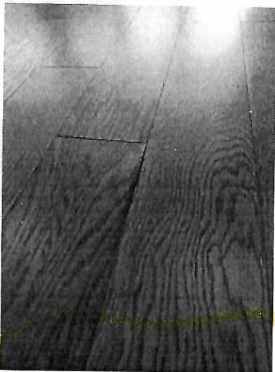
This plank is slightly bowed up this is where the front hallway opens into the living room
