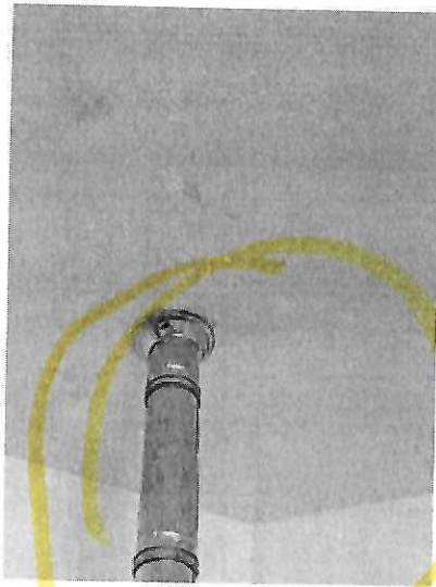
Minor tape seam crack garage ceiling
