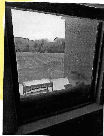
Back center living room window appears to be compromised
