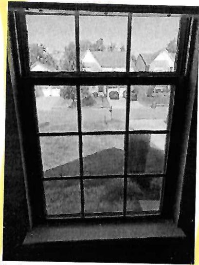
Bedroom 3 window upper pane showing signs of delamination, this is a cosmetic concern and does not affect the performance of the window.
