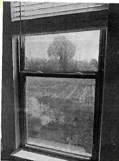
The right rear dining room window upper pane, has delaminating film.
